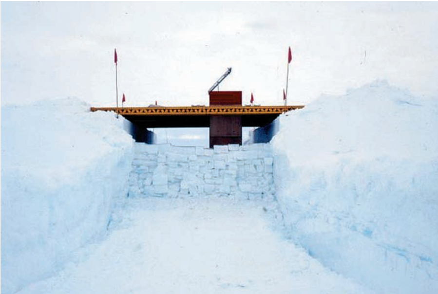
Fig. 3: Closing an open trench of the geomagnetic observatory successively by erecting walls of snow bricks and filling up the outer trench with snow. When the trench is completely closed the entrance shaft will be the only access into the observatory.
