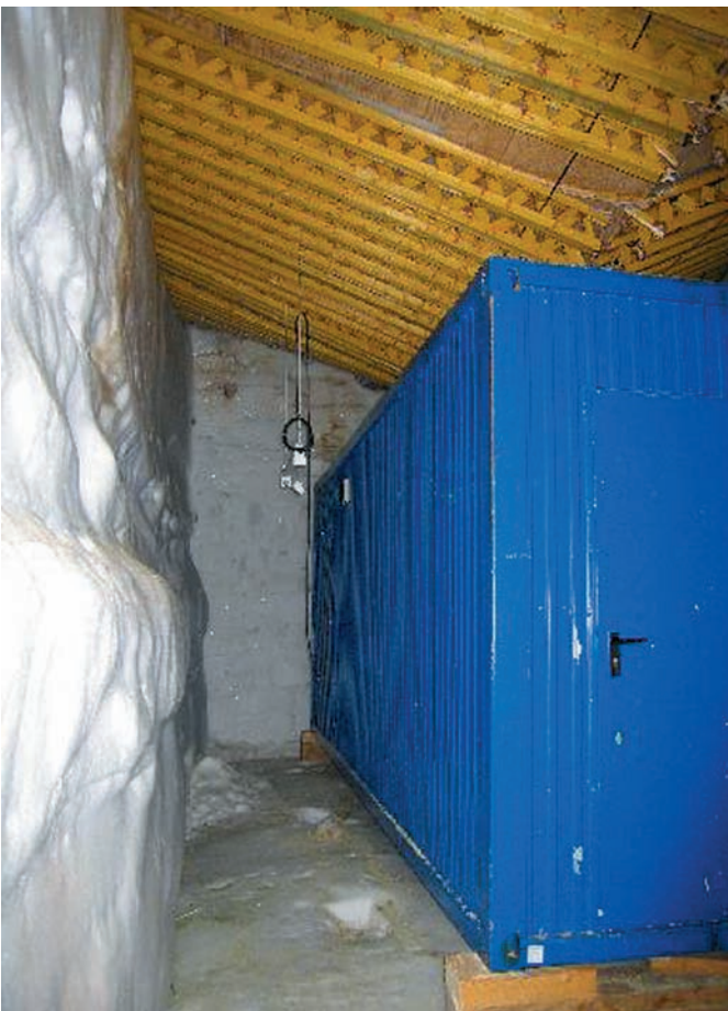
Fig. 4: Inside the closed seismic observatory in austral summer 2006. The wooden support beams of the roof had broken already some years before, but the snow masses above the roof have sufficient self-supporting strength against any sudden collapsing. The snow masses are only gradually, but steadily sinking with time. However, this observatory cavern was closed in 2003 and the equipment installed in the I27DE infrasound station.
