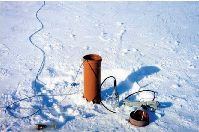
Fig. 8: Data acquisition units for the seismographic array are installed inside a container. Solar panels at the walls and on the roof recharge the batteries. Digital data are transmitted to NM-II via an UHF radio link (top). The 1-Hz Mark L4-C seismometers and a pre-amplifier are installed inside plastic tubes. Thus, seismometers and electronics are accessible at any time and can easily be recovered again (bottom).
