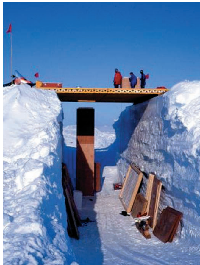
Fig. 2: Construction work at the geomagnetic observatory at NM-II. The w-golden roof is already finished and the entrance shaft is partly erected. Leaning against the side-walls of the trench are the plywood elements for the non-magnetic hut wherein later the sensors are installed. The height from the bottom to the roof is c. 7 m.
