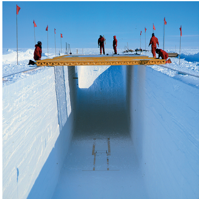
Fig. 14: Drill and science trench under construction: After the trench was excavated, it was covered with a wooden roof. The roof rests on wooden beams on top of compacted snow (see Fig. 13). On the ground of the six metres deep trench one recognizes the wooden foundation for the winch and the drill tower. (Photo H. Oerter, January 2001).
