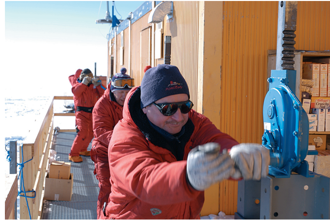
Fig. 11: Jacking up of the platform of Kohnen Station by winches mounted on top of the extended pillars. Each synchronous turn of the winches lifts the platform by three millimetres. (Photo H. Oerter, 18 01 2008).
