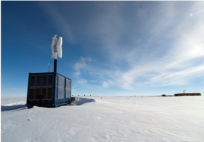
Fig. 29: Container with the automatic aerosol sampler inside at Kohnen Station (background right). The air intake is on the roof. Solar panels on the outer walls and the wind generator provide the needed electrical power for year-round charging of the batteries. The container had not been moved during the past two years. (Photo H. Oerter 11.01.2008).
