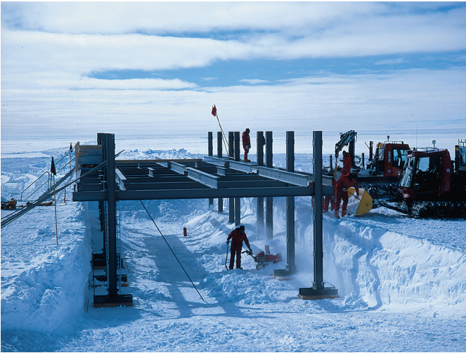
Fig. 10: Kohnen Station under construction. The excavation for the 16 pillars and the steel platform was 2 m deep (cf. Fig. 9). Some of the footplates under the pillars are already covered with snow by means of a small snow blower. Later the whole excavation was filled completely with snow. (Photo H. Oerter, 06 01 2000).
