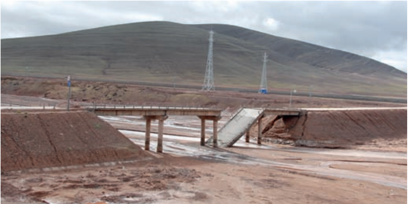
Figure 18: Permafrost thawing near the base of the support pillars caused this bridge on Qinghai-Xizang Highway in Tibet to collapse (photo: Tingjun Zhang).
