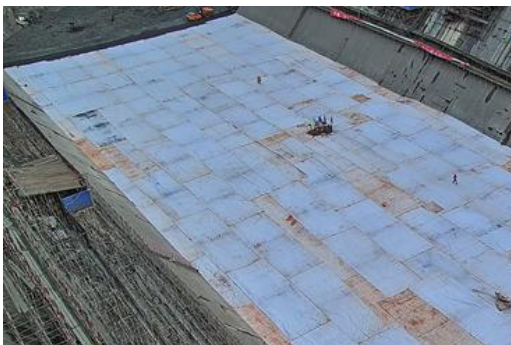
Figure 4. Dam core covered with thermal insulations made by nonwoven geotextile and LDPE geomembrane.
