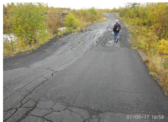
Fig.1. Deformation of roads during permafrost retreat.
