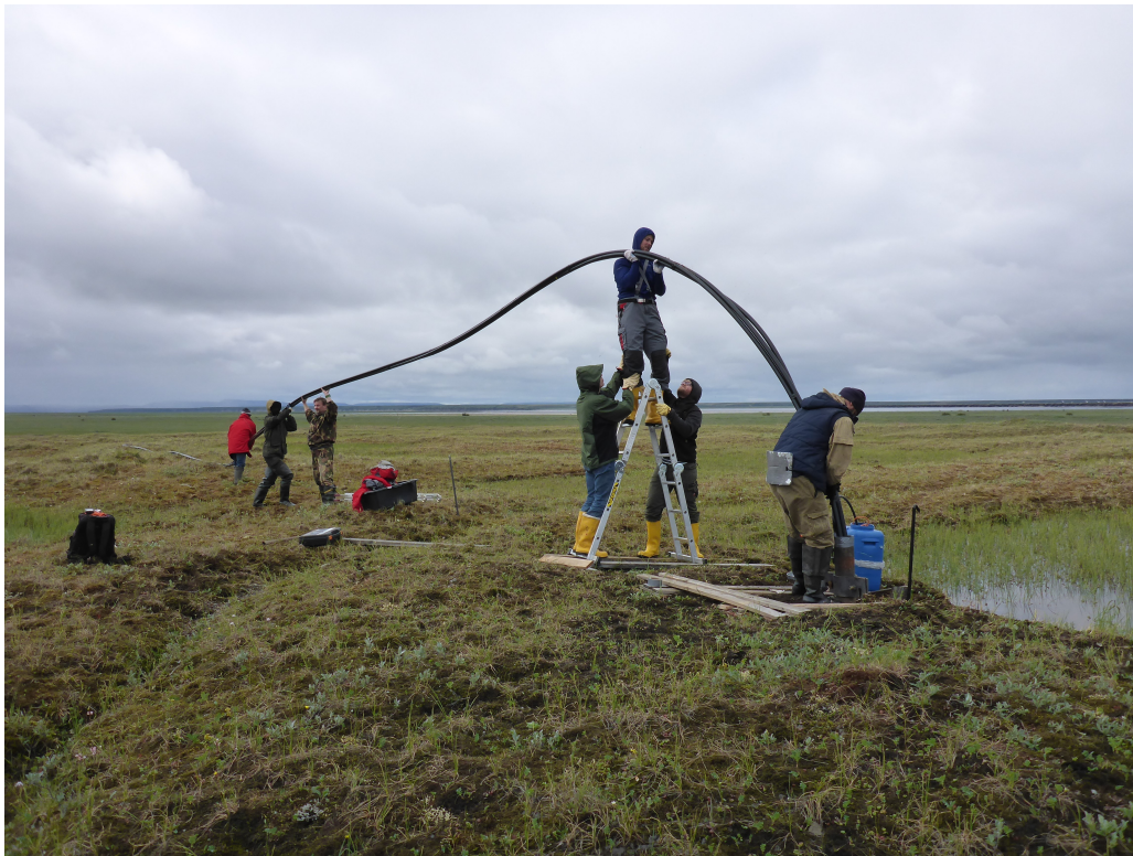
Figure 2.2.3: Installation of the new borehole on July 9 th , 2018. Photo by Niko Bornemann
