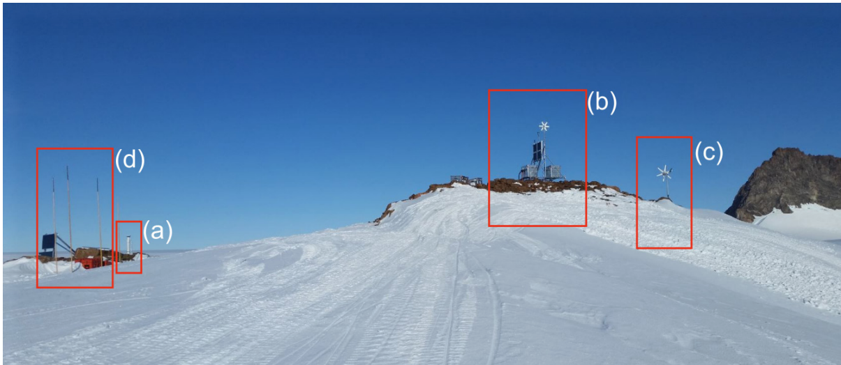
Fig. 4.18.4: Test installation of GNSS site KOP1 at Weigel Nunatak with (a) GNSS antenna on top of pillar, (b) solar panel, first wind generator and box containing receiver and batteries, and (c) second wind generator. The collocated seismometer station (AWI) is situated at (d).
