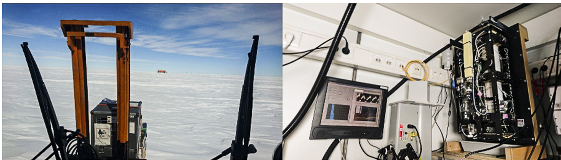
Fig. 4.11.1: Transport of the CCN instrument to SPUSO (left) and after finalized installation and connection to the same inlet as the other aerosol instrumentation (right)
