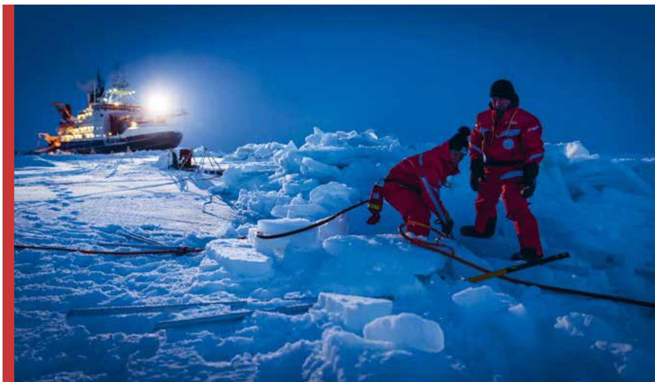
Two researchers dig out a power cable that was buried when a pressure ridge formed nearby.
