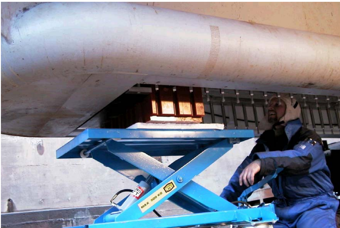
Figure 5 Transducer element installation on “Commander Jack”
