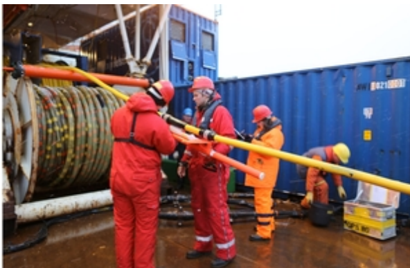
Fig. 1. Fixing a depth controller unit onto our streamer (yellow). This unit is remotely controlled from the seismic recording lab during the survey. (Photo: A. Bublitz/YUoT).
