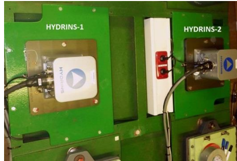
Figure 3-5: Installation of the HYDRINS-1 and 2 in the Gravity Room of RV Polarstern (AWI)
